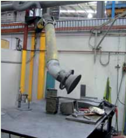
Fixed extraction unit assists in removing exposure to fumes, the unit is manoeuvrable to ensure fumes are taken away from the welder at all times.
