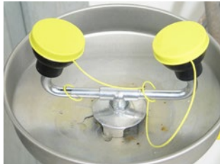
Figure 2. Eyewash with protective covers.
